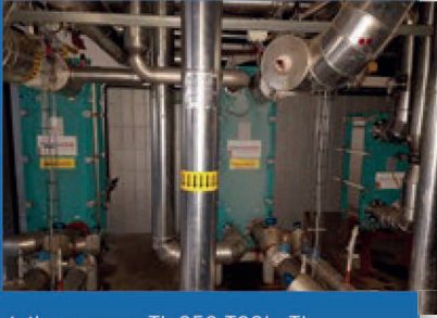
▲ thermowave TL 250 TCGL, TL 500 TCGL and TL 850 KCIL plate heat exchangers form the interface in each case between the circuits for ammonia and green beer.
