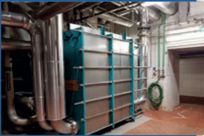
▲ In Tychy, wort is cooled from 99 °C to 10 °C using five thermowave TL 500 TCGL plate heat exchangers with a combined plate heat exchanger capacity of 32 MW.
