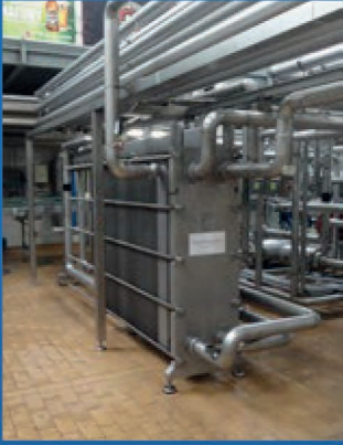
▲ A thermowave TL 500 FCGV unit, which boasts approx. 93 % heat recovery, is used as a pasteuriser for the high-temperature, short-time (HTST) flash pasteurisation of the beer for 15 to 30 seconds.
