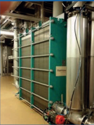
▲ A thermowave TL 850 KBKL unit with a heat exchanger capacity of 6.5 MW heats up over 200 m 3 of wort per hour from 72 °C to 98 °C. In the counterflow, 100 °C hot water is cooled as part of this process step down to 78 °C.
