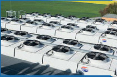
▲ AGVH-type Güntner FLAT Vario condensers each with 595 kW/2,030 MBTU/h have been designed as special units due to building regulation noise specifications of 50 dB(A)/10 m (33 ft) in order to achieve the specified operating parameters.
