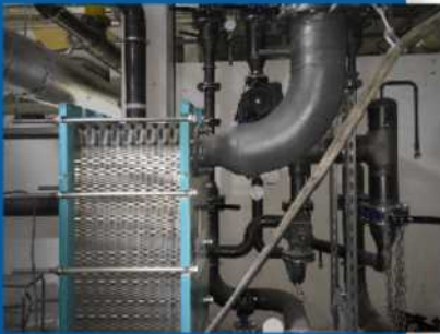
The thermowave plate heat exchangers are located at a depth of 12 metres below the 44,000 m 2 construction section which is the latest of the building ensemble.
