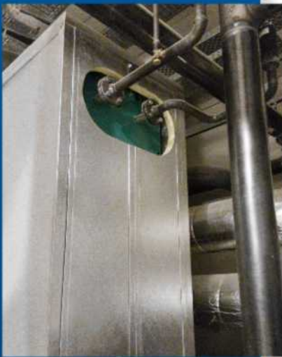
The German heating system regulation stipulates that plate heat exchangers are to be jacketed.
